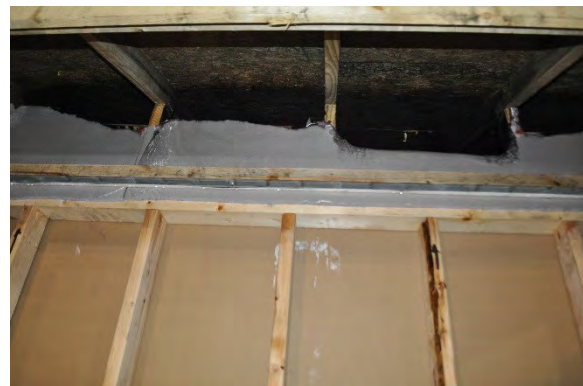
Figure 10. 39. View into the eaves after Attic Fire Experiment 4
