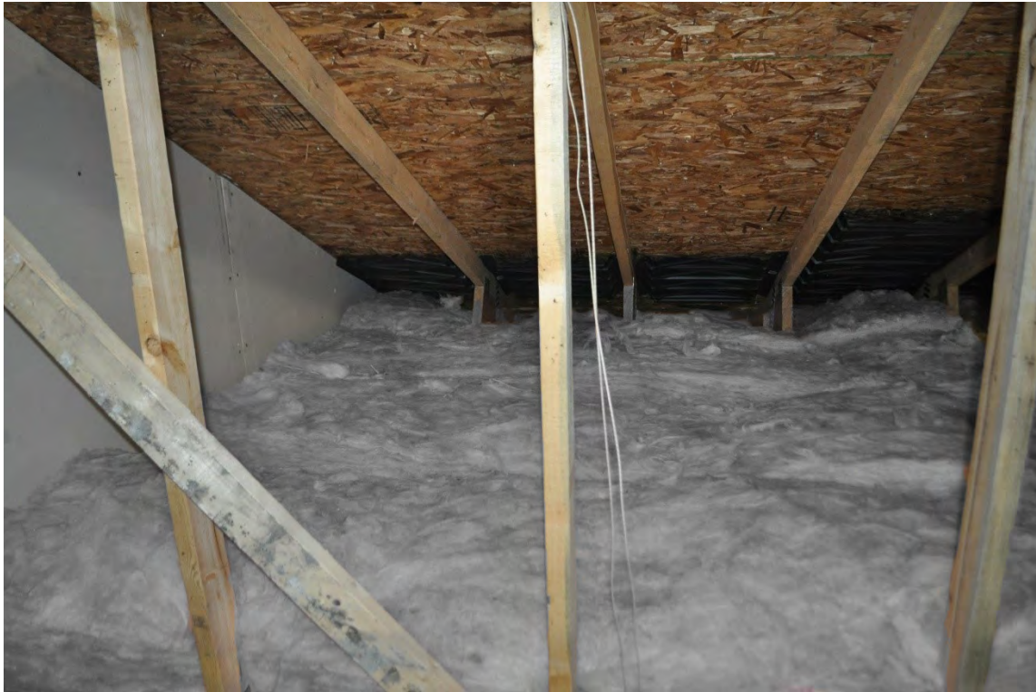
Figure 7. 11: Plastic Ventilation Baffles
