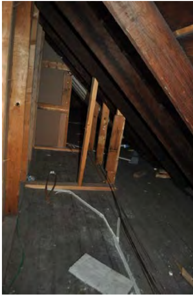
Figure 10. 52. Knee wall access showing difficulty of flowing water past the rafters.
